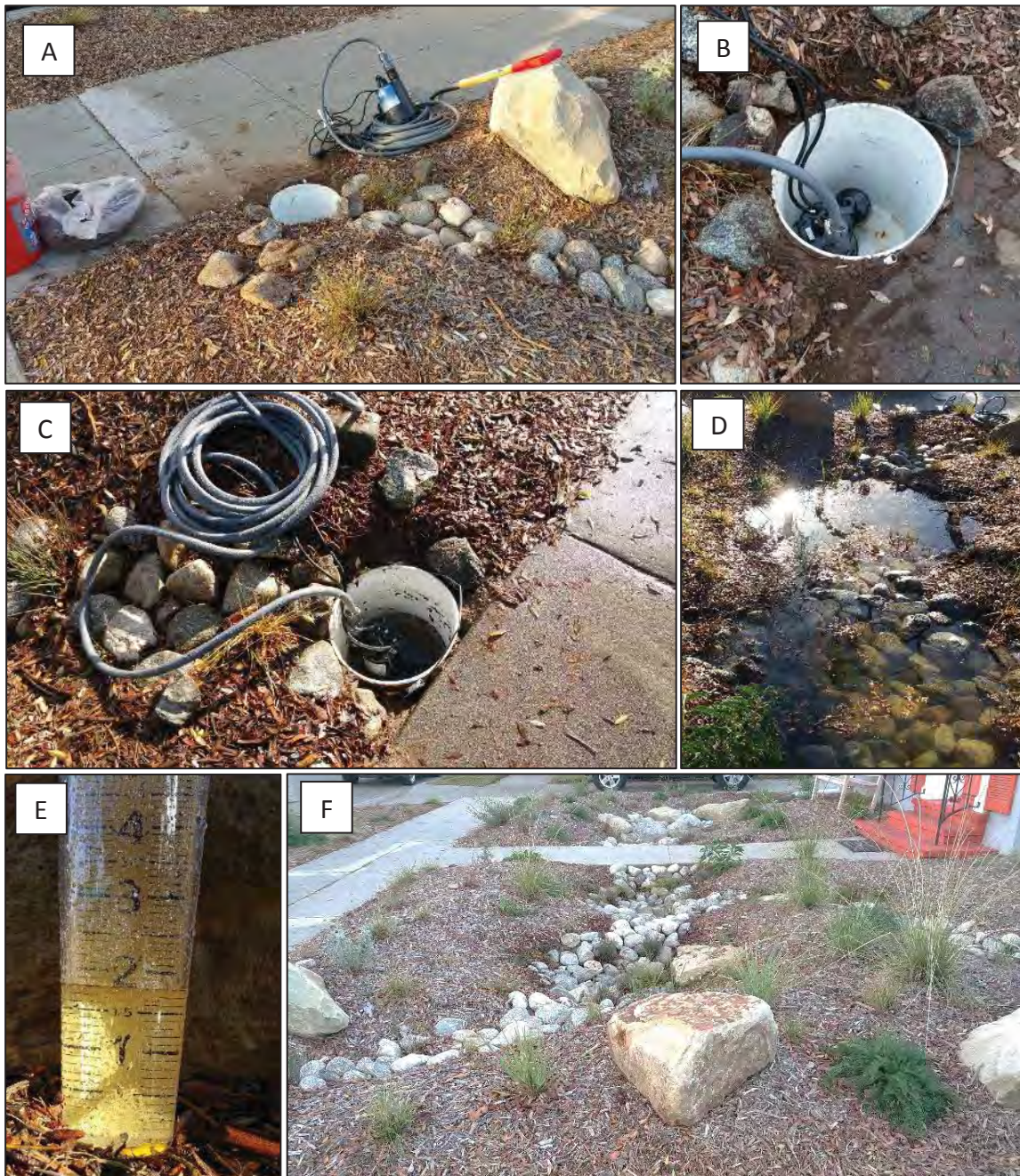
Figure 17. Post-implementation stormwater monitoring (Site 2, Wagner). Pre-storm installation (1/4/2016): (A) 5-gallon bucket installed at bioswale overflow; (B) automated pump, hose, and water meter to assess installed. Post-storm assessment: (C) Bioswale overflow monitoring post-storm (1/5/2016); (D) bioswale ponding (1/5/2016); (E) on-site rain gauge (1/5/2016); (F) complete bioswale infiltration (1/6/2016).
