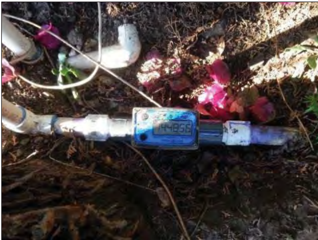
Figure 2. Photo of sub-meters installed at a residential property.
